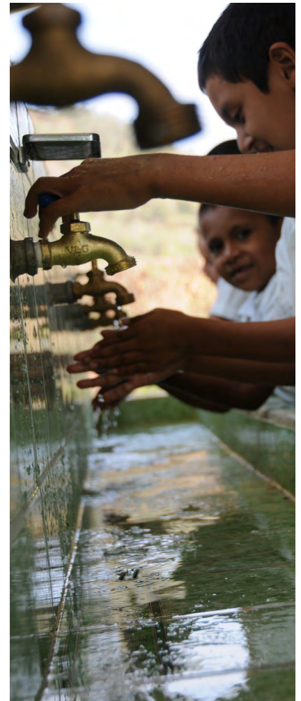
Above: At a SWASH+ school in Honduras in 2010, students have a ready supply of water for hand washing.
