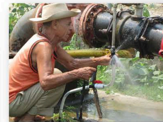
Mechanic working in Potrerillos, Honduras, fixing a water system leak. - Photo courtesy of Mark Taylor (2010)
