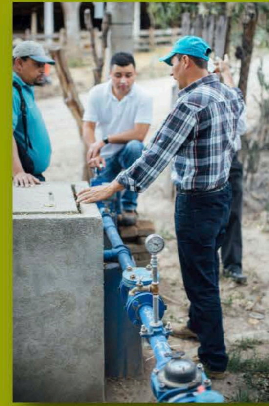
Community water system – water meter
