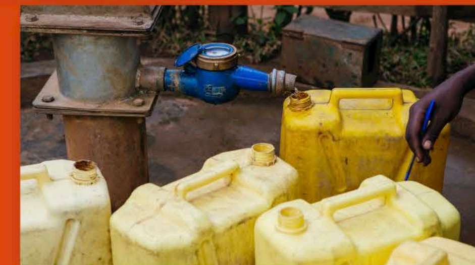
Water meter at a well
