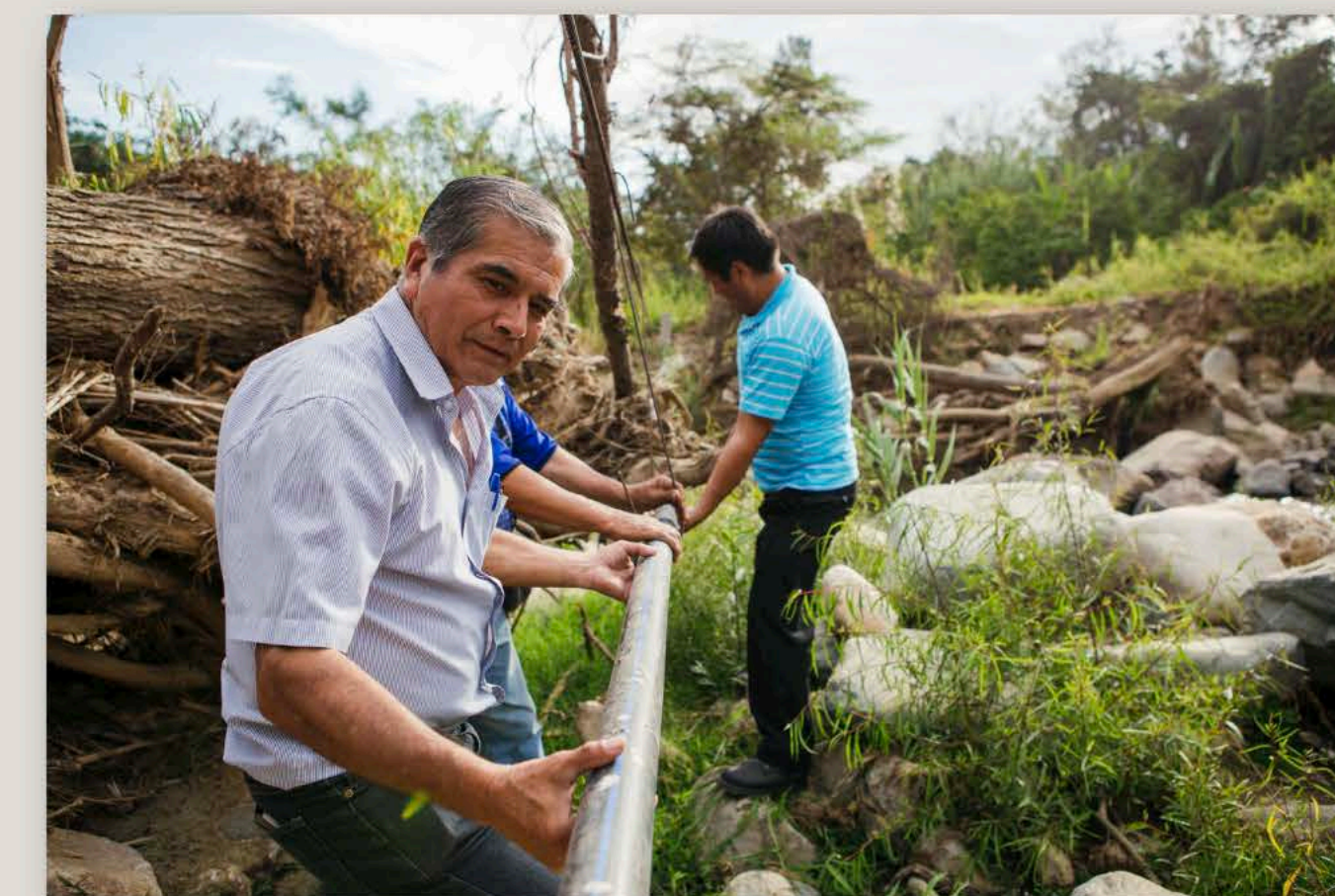
Repairing a water distribution system in Peru after El Niño storm in 2017
